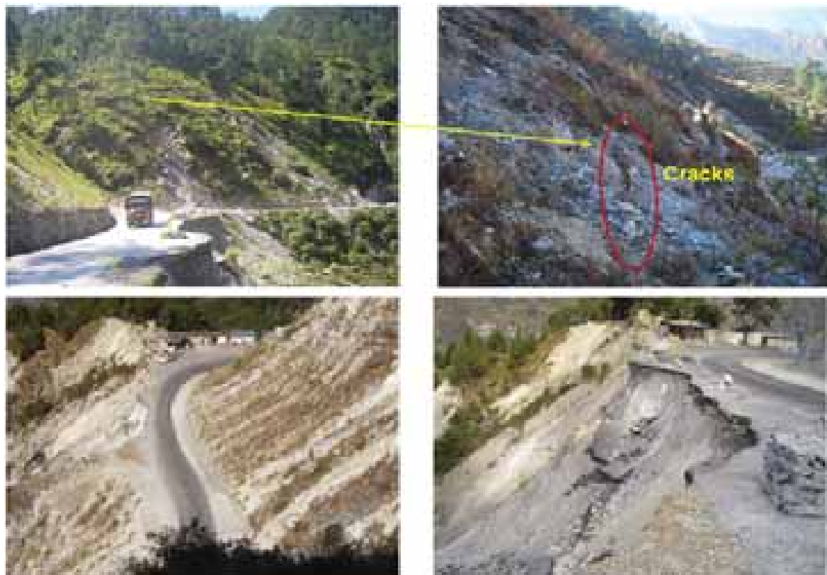
Fig.6: View of landslides
