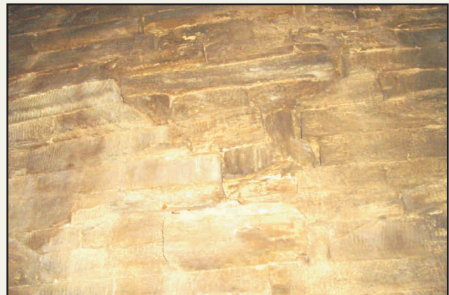
Indication of Settlement & Tilting
