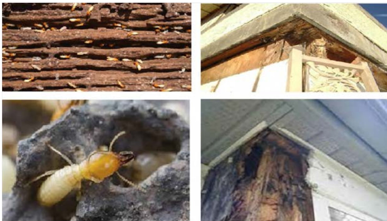
Fig. 1: Termite and its damage in buildings
