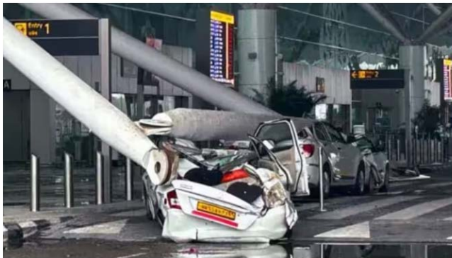
After Delhi Airport canopy collapse, government enlists CBRI to advise airport operators on structural safety.
